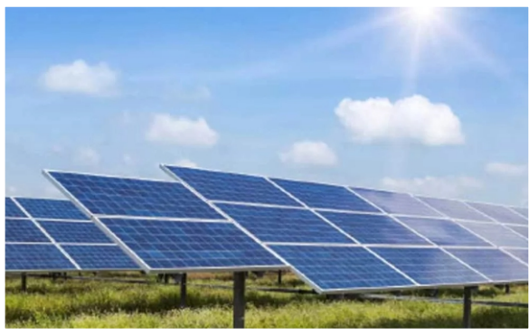
Solar Plant Nathra 2 MW
