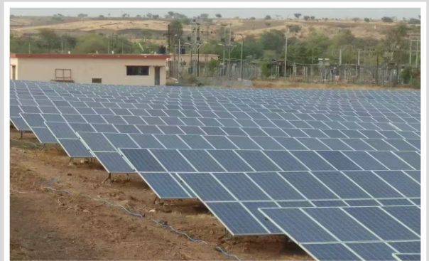
Solar Plant Project in Tuljapur Dist. Dharashiv
