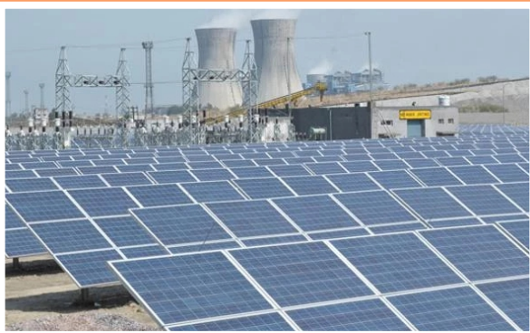
Solar Plant Parli Vaijinath 10 MW
