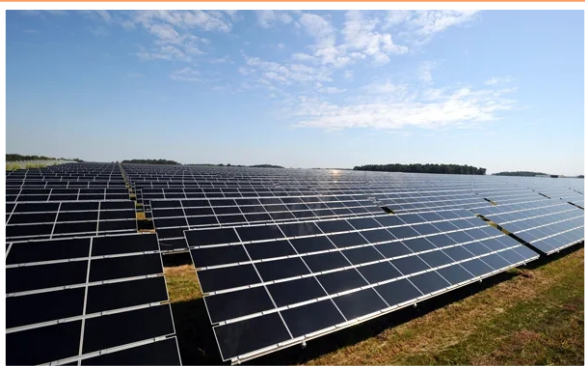
Solar Plant Ahmadpur 6.25 MW
