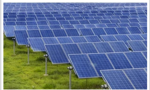
Solar Plant Project in Solapur
